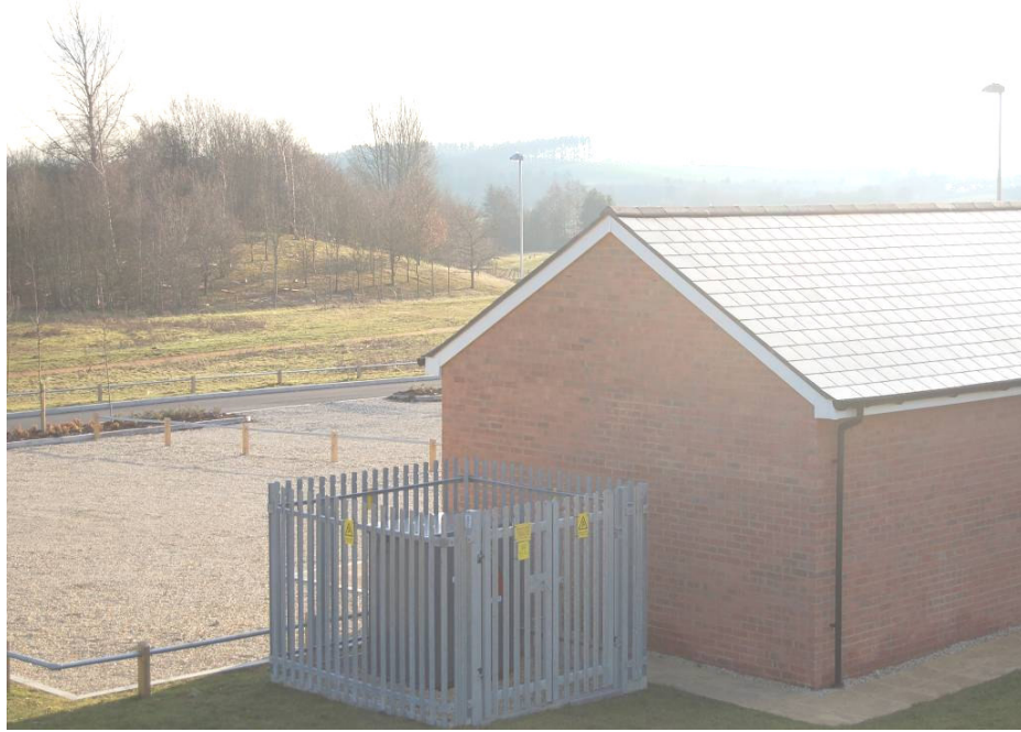
Figure 27 View looking south showing electrical sub-station against east elevation of store
